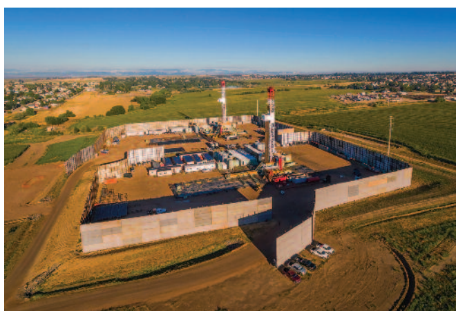
Temporary 32-foot sound walls enclose SRC Energy Inc.’s Evans pad in the D-J Basin, dramatically reducing noise and light output from wellsite operations. The two rigs finished drilling 22 horizontal wells on the pad last year, including 13 ‘long-length’ laterals averaging 10,000 feet and nine ‘extended-length’ laterals averaging 12,000 feet. Ahead of the horizontal drilling program, SRC plugged 27 legacy vertical wells on the Evans spacing unit and reclaimed
